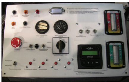
Central Control Console
